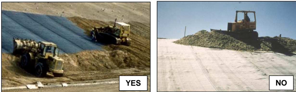
Figure 15. Cover soils should be pushed from the bottom of the slope up, not from the top down.
