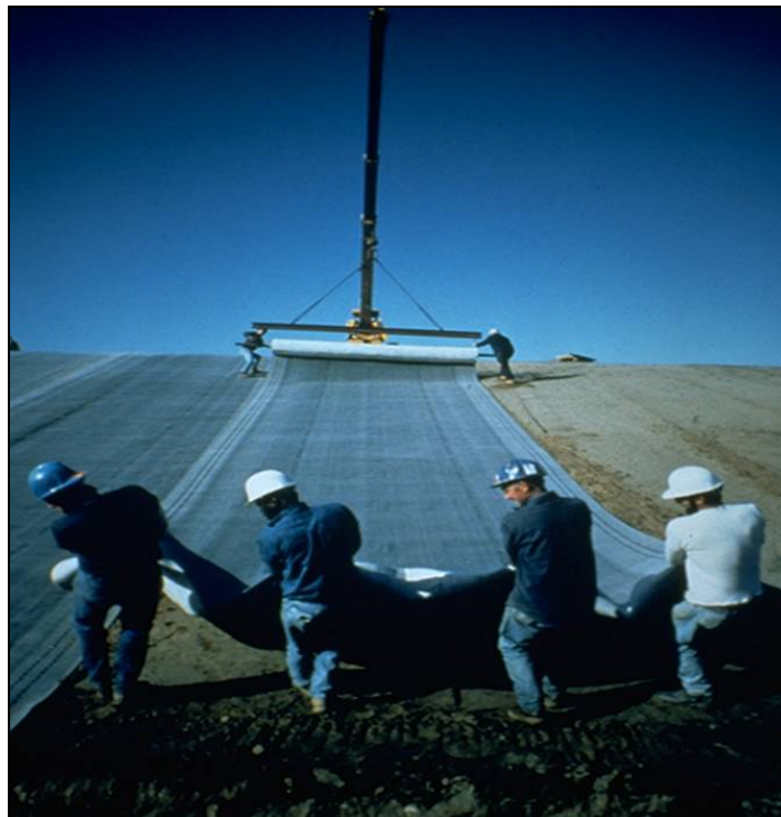
Figure 7. Manual deployment down a slope. It is generally not possible to pull the liner upslope.
